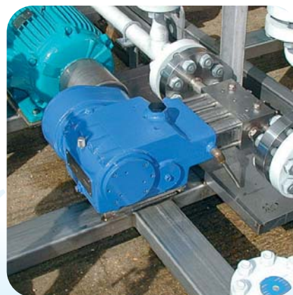
HP5650 pumping Arctic diesel
